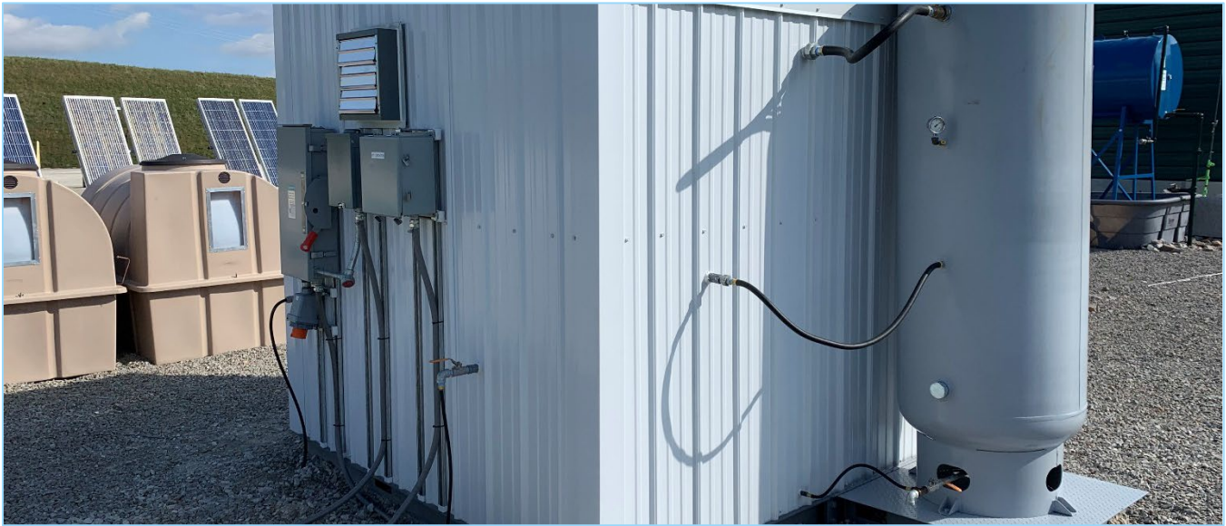
The compressed air system is housed in a shed, which helps prevent freezing in the winter.
