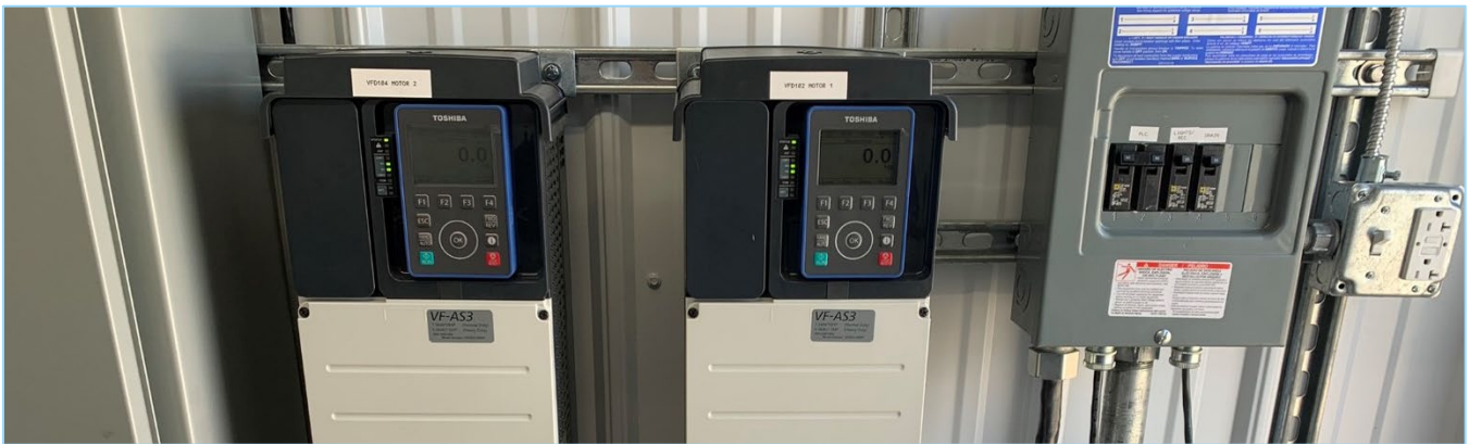
Motor drives regulate the compressor speed to match the air needs of the pad.
